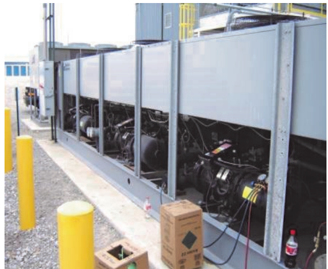
(4) CSH6563-60-4PU Screw Compressors (60 Horsepower)
